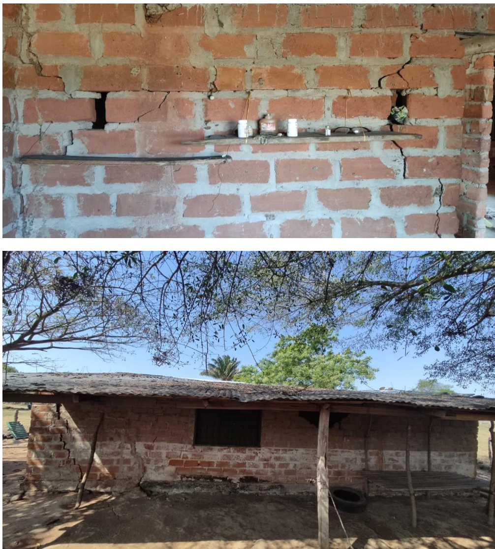
Figure 6 & 7: Possible cracking of housing. Photographs by author.
