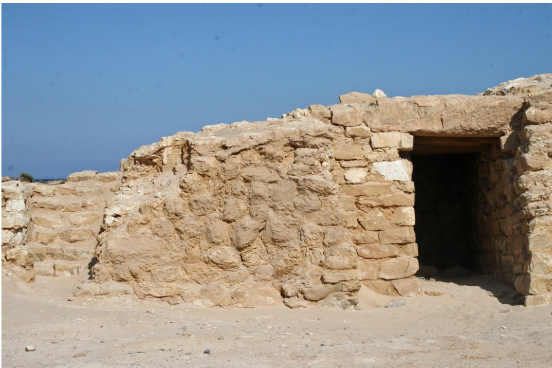
Figure 18: 2008 view of the fort's western interior with the stairway, retaining wall, and the unblocked/open eastern end of the entry passage (Photograph: P. Carstens)
