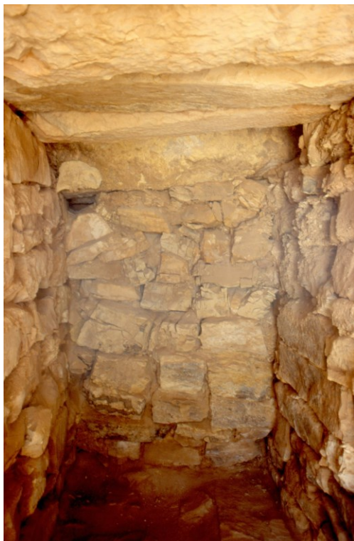
Figure 12: View of the 1+ m wide stone blocking sealing the western end of the fort's original entry passage (Photograph: P. Carstens)
