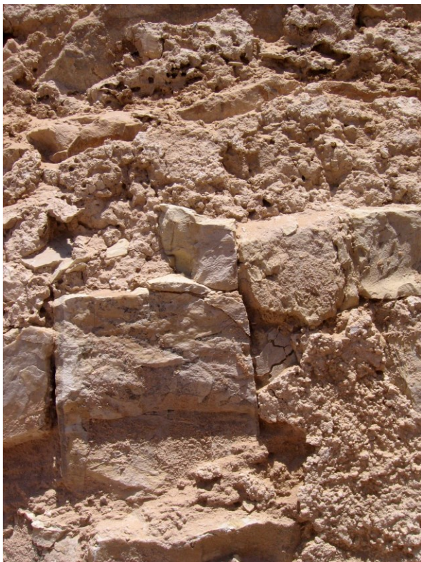
Figure 14: Detail of the salt encrustation on the stone and mud blocking sealing the exterior face of the fort's original western entryway (Photograph: G. Mumford)
