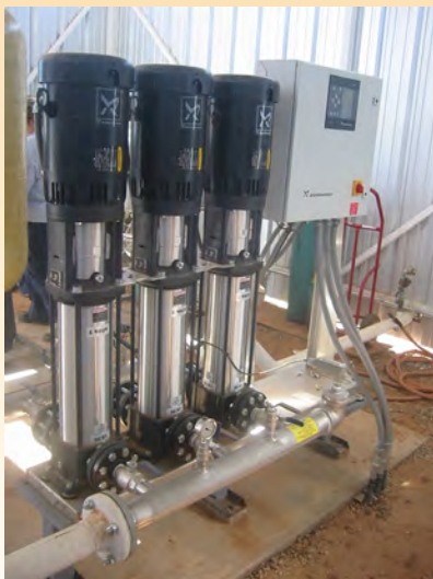
An arsenic treatment system on the Tohono O’odham Nation // Photo courtesy: Seldo Villegas
